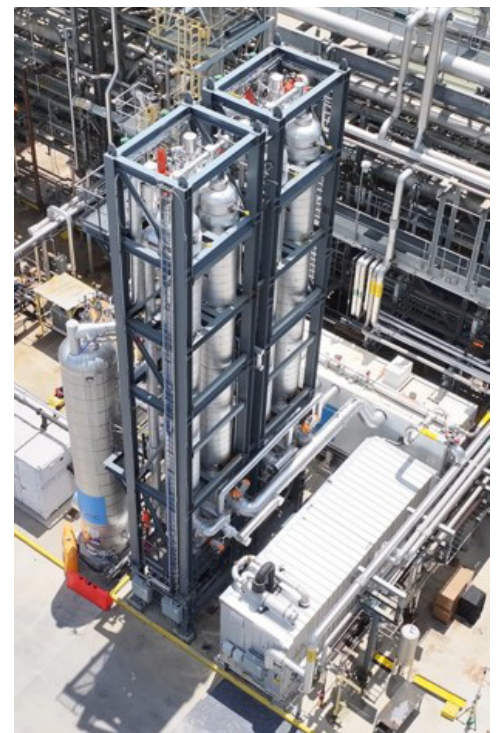
The FrostCC™ system installed at the NCCC in Wilsonville, Alabama. (Photo: Business Wire)
