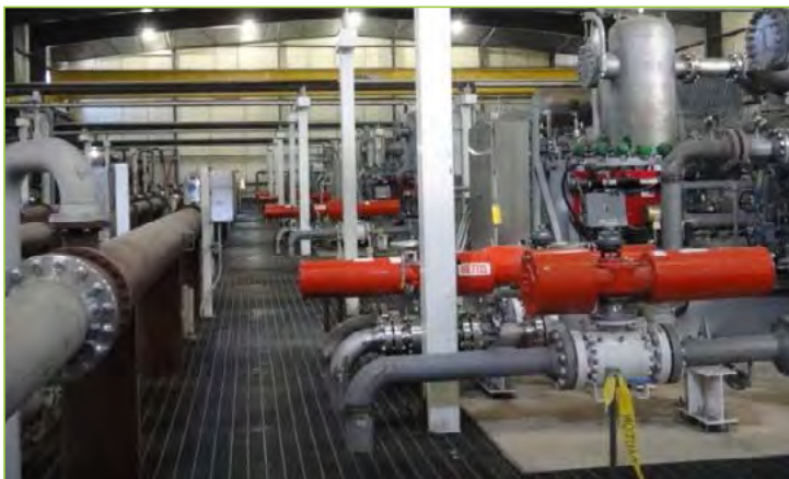
Inter-Stage Piping in Compressor Facility (Courtesy of Archer Daniels Midland Company)
