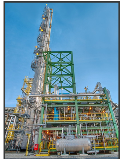
Linde-BASF 1 MWe Pilot Plant at NCCC
