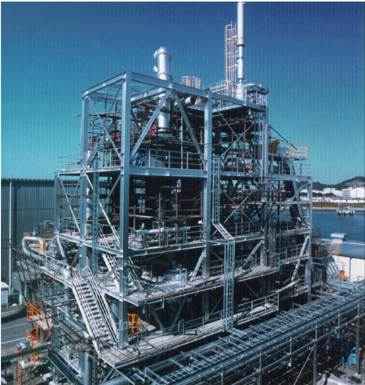
Fig. 9: The 20 tpd HTW waste gasification plant at Nihma, Sikuku, Japan
