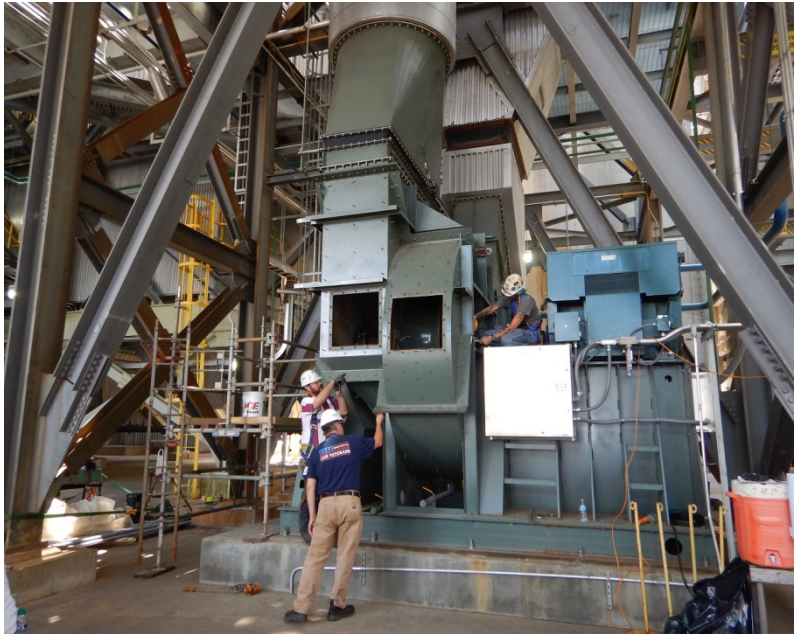
Flue Gas Blower
