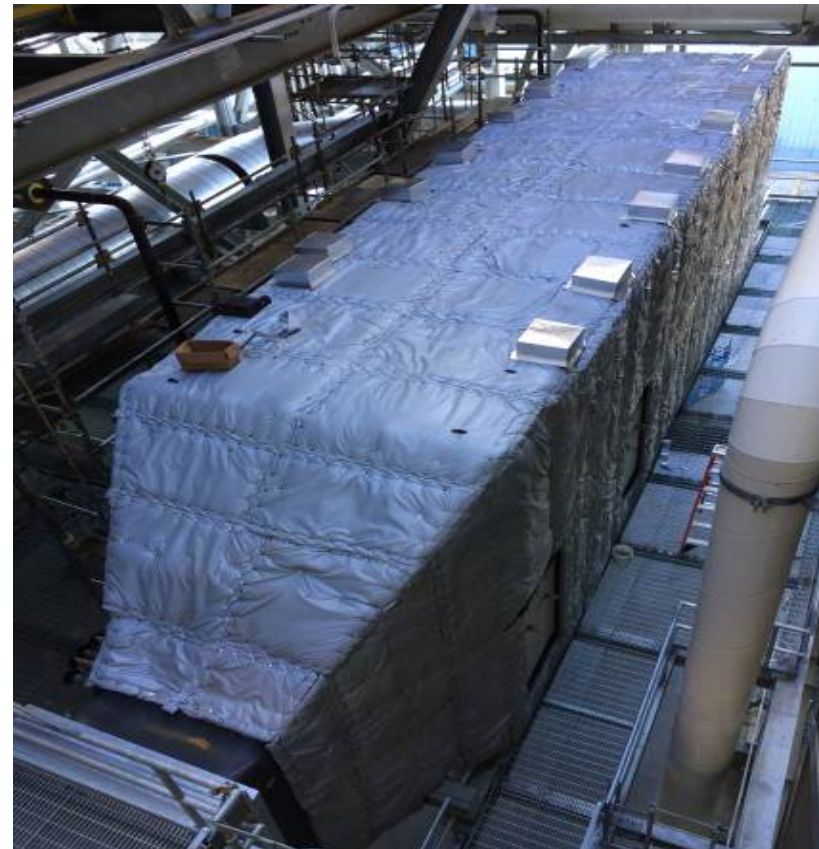
Flue Gas Cooler
