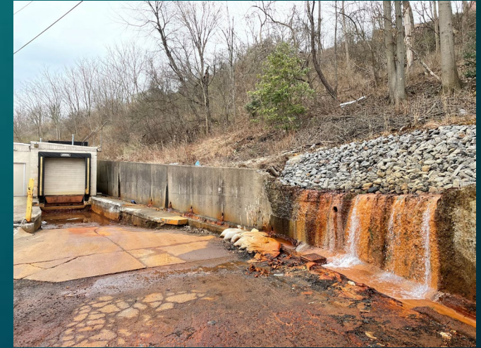
AML damage in West Newton, PA
