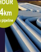
1.4m dia pipe @100bar
