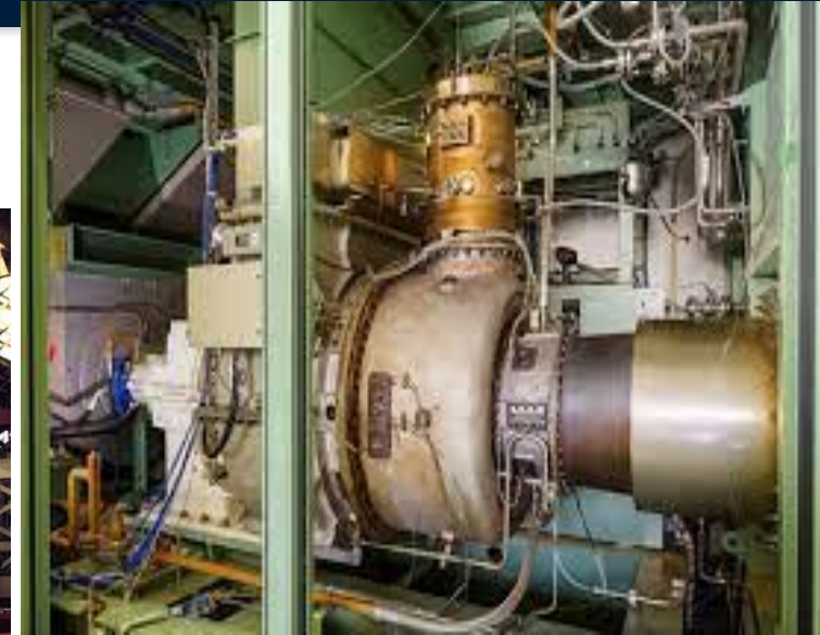
IHI Ammonia Gas Turbine- 100% NH 3 [ https://www.ihi.co.jp/en/all_news/2022/resources_energy_environment/1197938_3488.html ]
