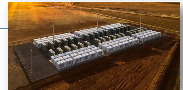
Grand River Energy Center - BESS ~200 MW Battery Energy Storage System (BESS)
