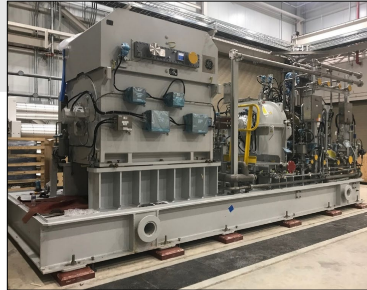
Main Compressor system and drive
