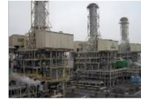
Waste Heat Recovery
