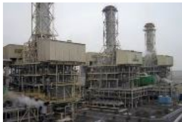
Waste Heat Recovery
