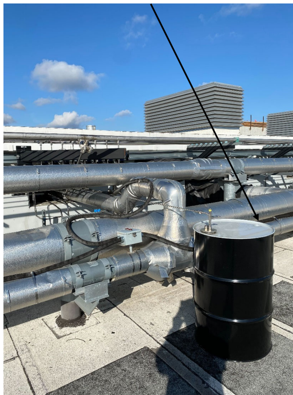
Vent port uncapped
