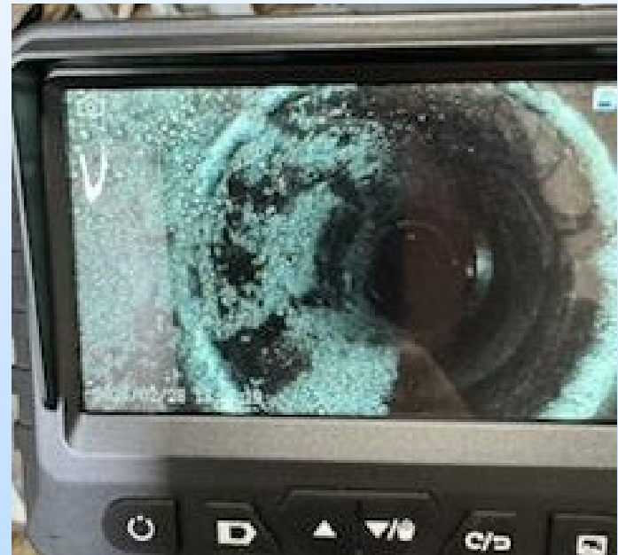
Debris seen in discharge pipe
