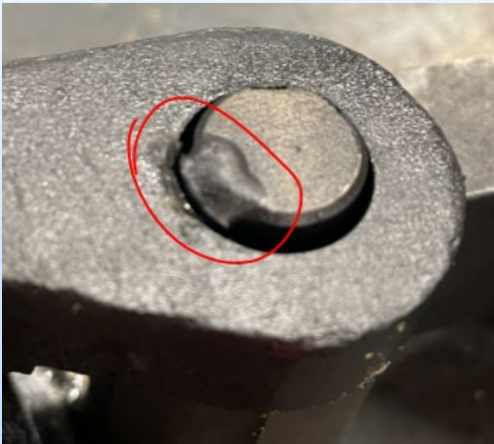
Damaged swing check-valve
