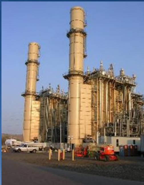
Natural Gas & Hydrogen Combined Cycle Power Plant
