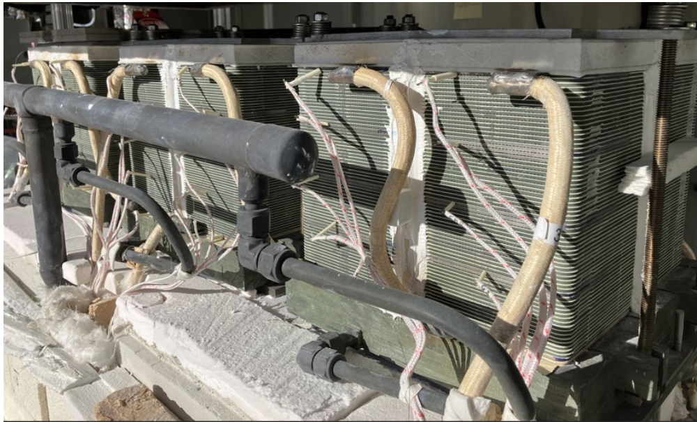
OxEon stacks with voltage taps and current conductors
