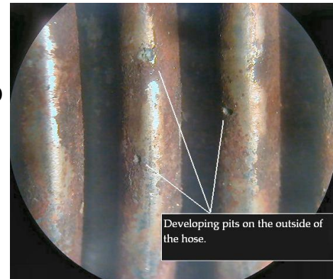
Example of chlorine corrosion on heat exchanger pipes 2
