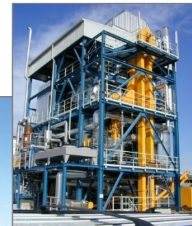
Güssing, Austria—heat and power production
