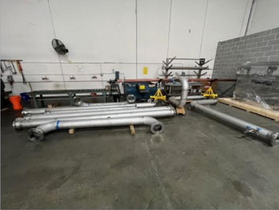
Large bore SS piping
