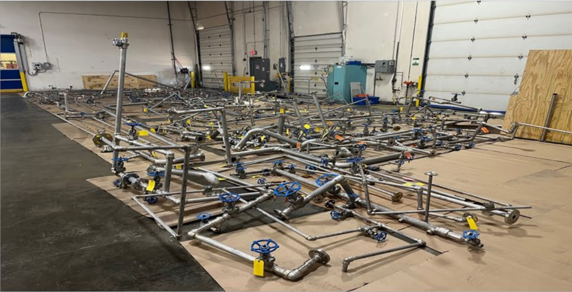
Various SS valves and piping
