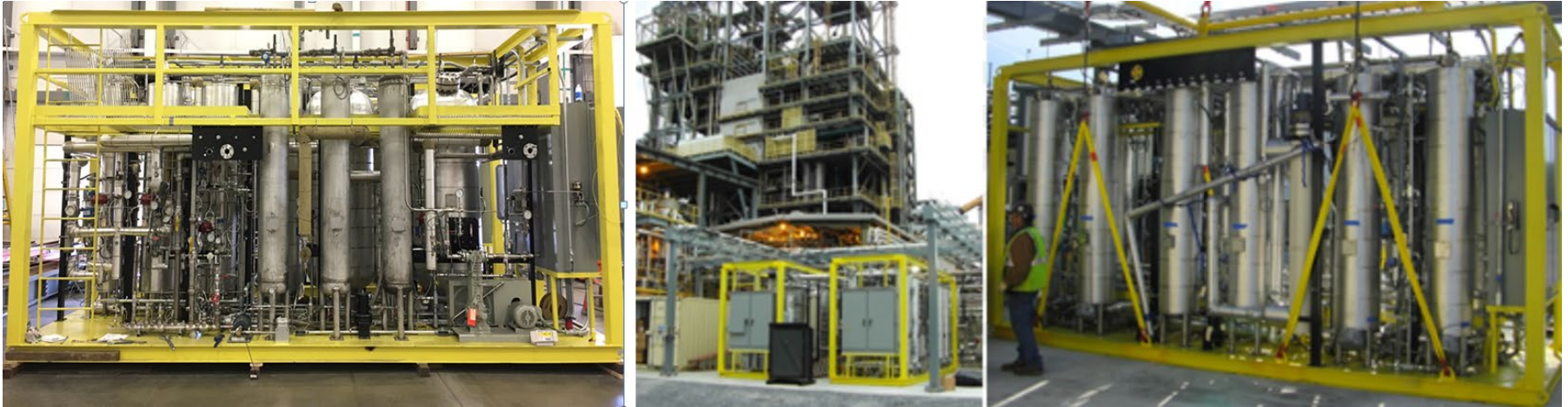
TDA 0.1 MW pre-combustion carbon capture unit installed at the National Carbon Capture Center
