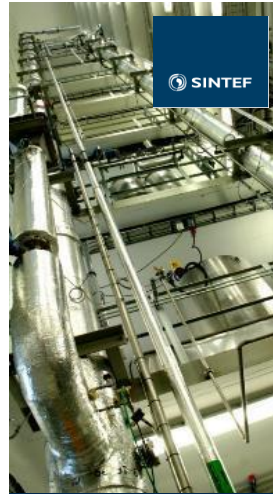
SINTEF Pilot Testing at Tiller Plant (2015-2018)
