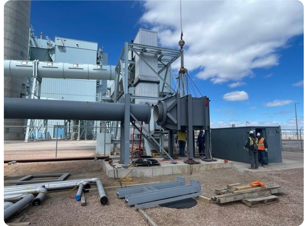
ITC tie-in and transition section
