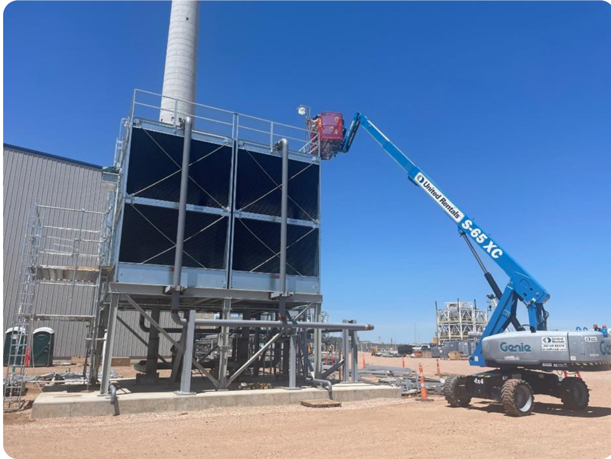
Electrical connections to the cooling tower
