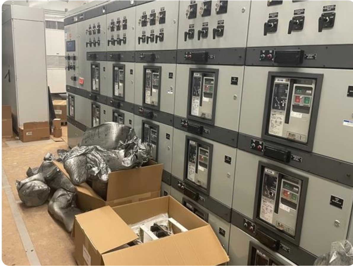
PDC Interior – electrical switchgear and motor controllers
