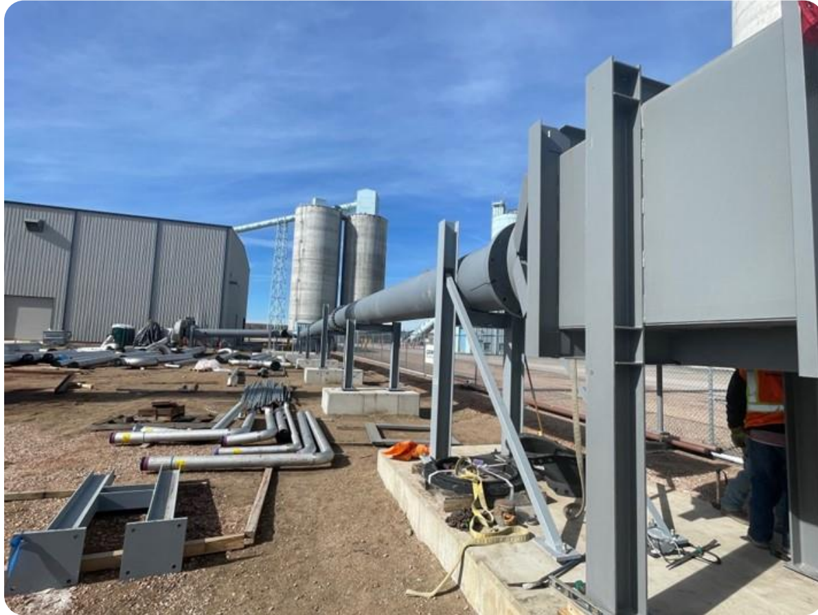
Duct run from ITC tie-in to the flue gas blower
