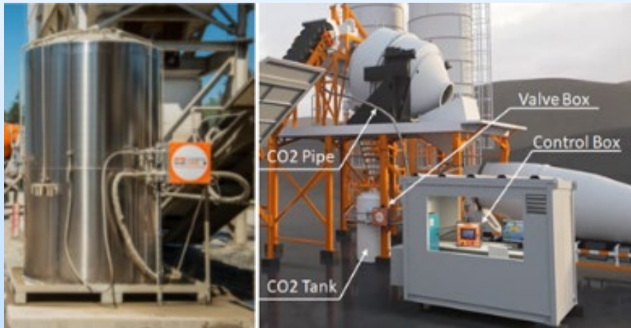
CarbonCure's CO 2 Dosing Tank and Utilization System
