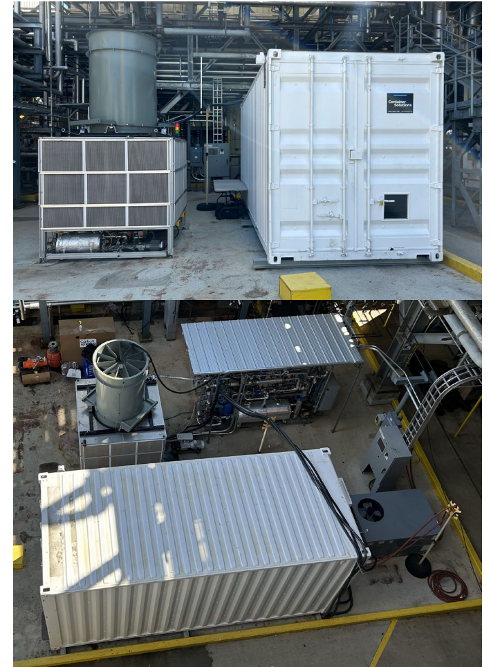
SN1 + Liquefaction at NCCC
