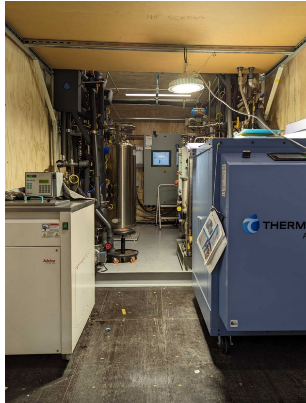
Liquefaction Skid Operating Inside Container
