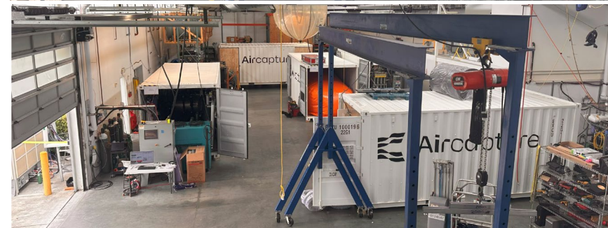
8x DAC-100 + Supporting BOP Skids for Project Hajar, June 2024 >50% cost reduction from SN-1
