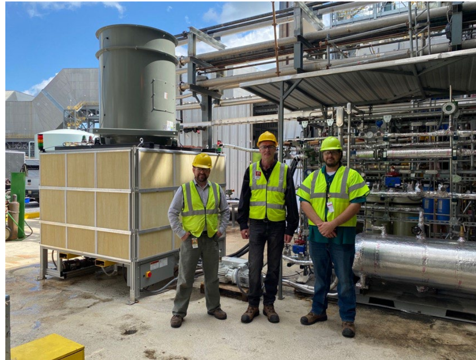
Aircapture Commissioning Engineers at NCCC
