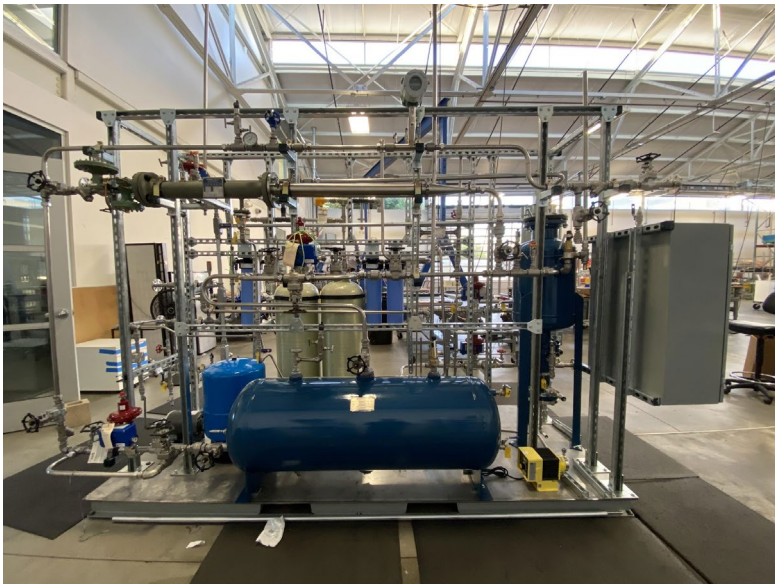
Completed Multi-mode Heat Integration Skid
