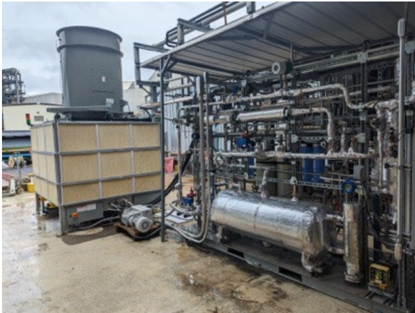
DAC Skid (left) Heat Skid (right)
