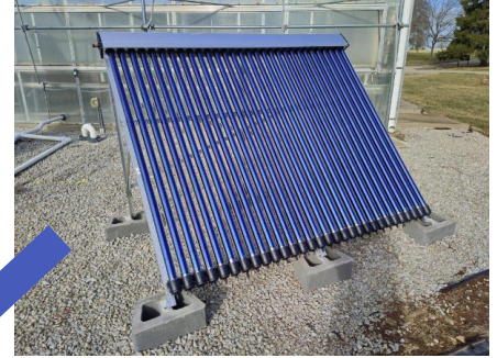
Solar Water Heater
