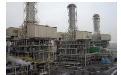
Waste Heat Recovery
