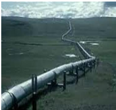
Pipelines: Monitor corrosion, gas leaks, T, acoustics to predict/prevent failures. NG, H 2 , CO 2 .
