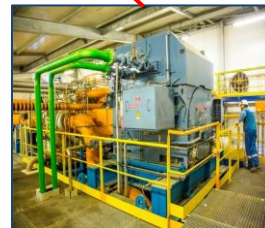
PSA tail gas & CO 2 product compressors
