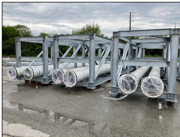
Pipe racks and cooling water piping delivered to site
