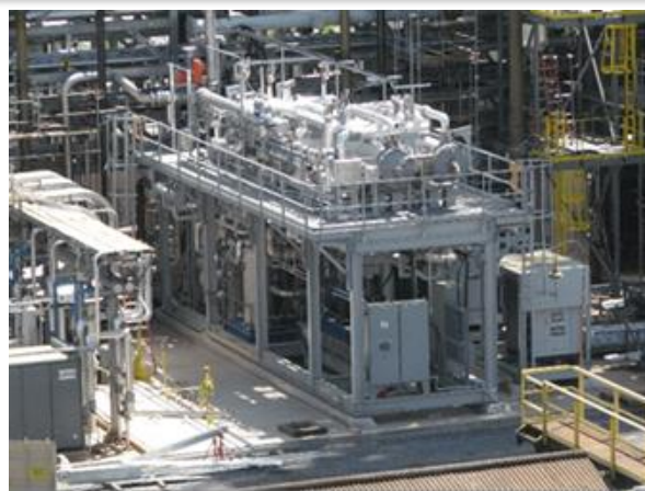
Existing MTR Membrane Module
