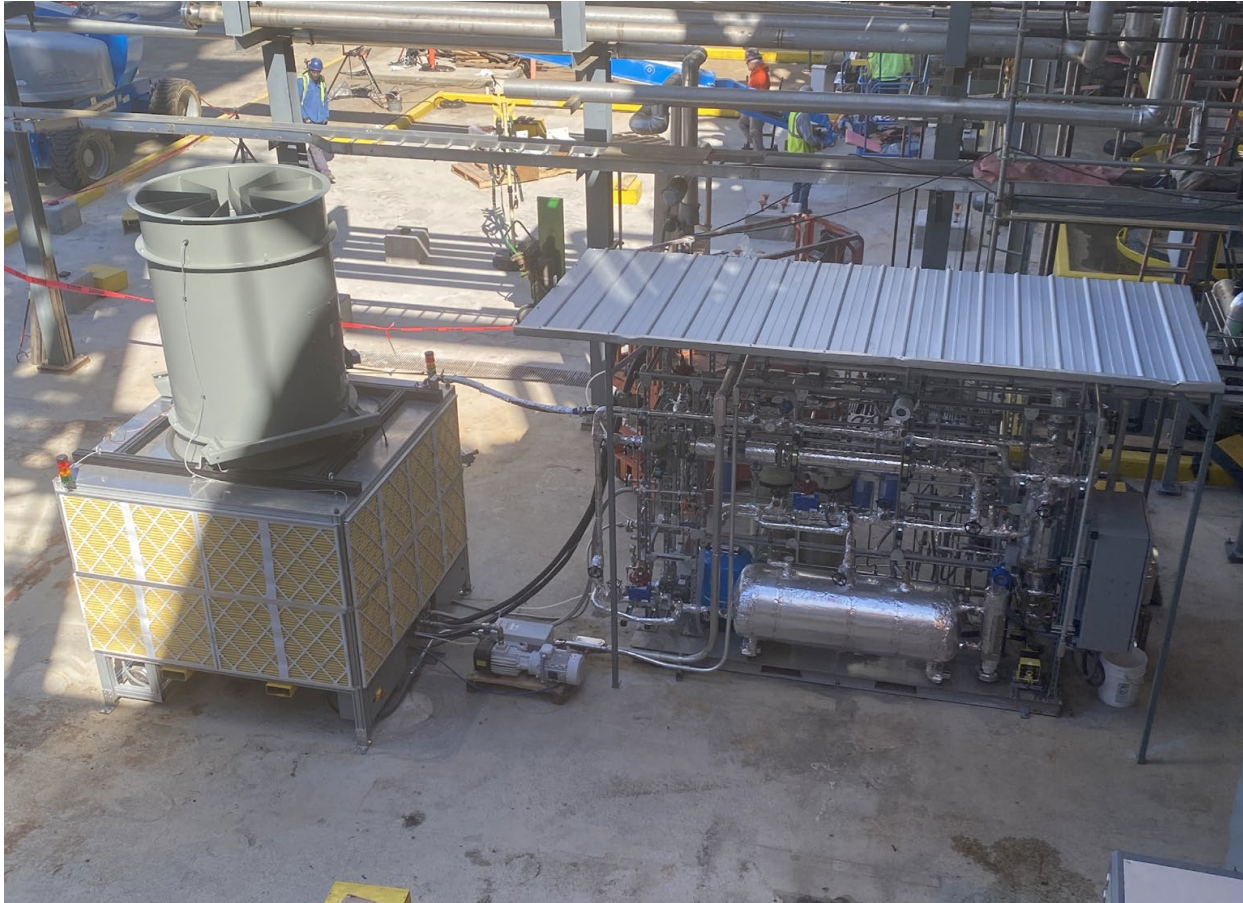
SN1: NCCC, Wilsonville, AL: March 2023 to present
