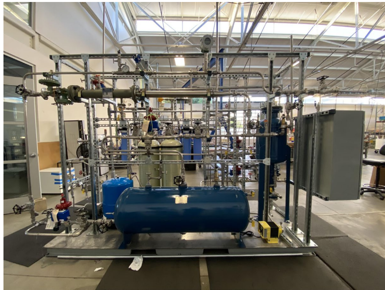
Completed Multi-mode Heat Integration Skid
