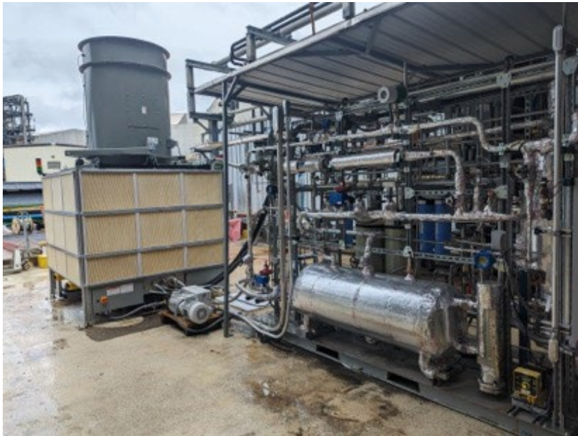
DAC Skid (left) Heat Skid (right)
