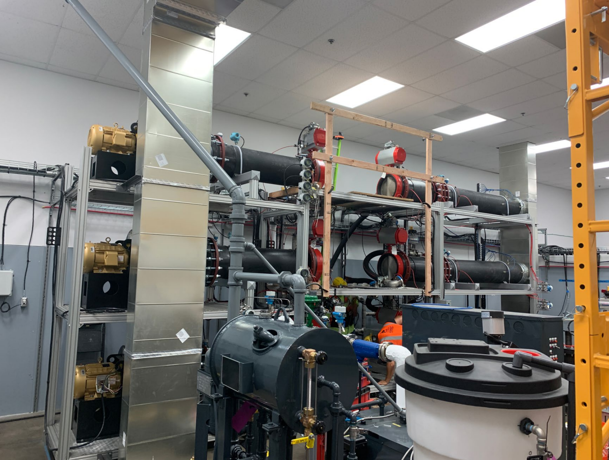
Test plant built with 3 independent parallel lines for DAC cycling:
