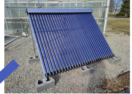
Solar Water Heater
