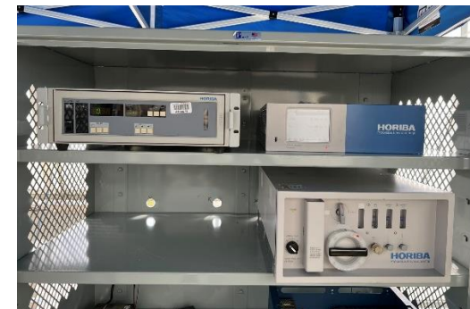
Gas Analyzer and Sensor Cabinet
