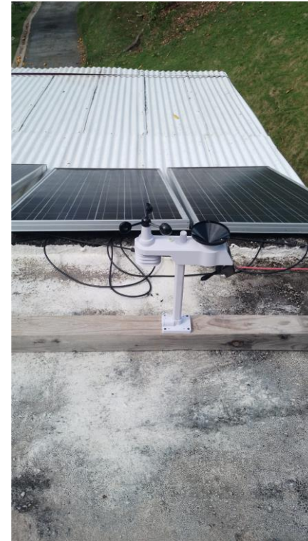
Fig. 3 Weather Station on ceiling
