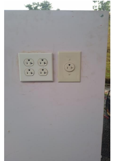
Fig 6. Outlets for electrical equipment
