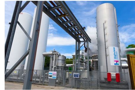
Highview, liquid air energy storage
