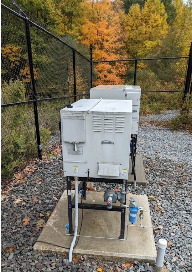
Wellhead Controls in New York
