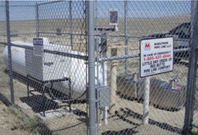
Cathodic Protection Site in Wyoming
