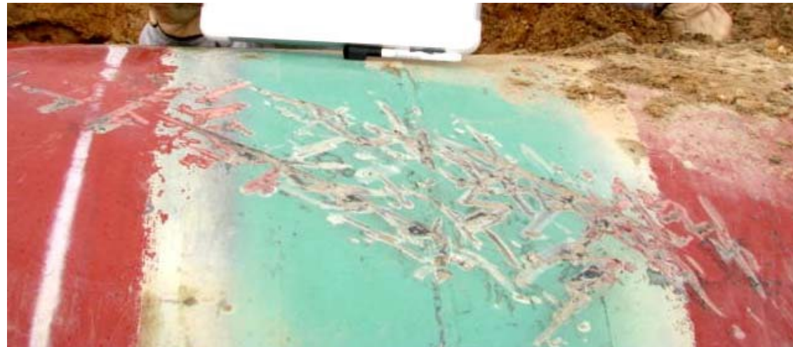
Construction damage of girth weld coating found by DCVG Survey during pipeline operation
