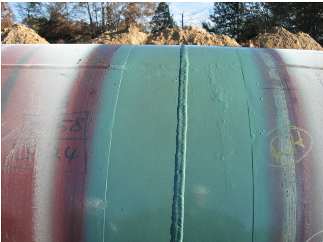
Field coating applied over dirt/debris
