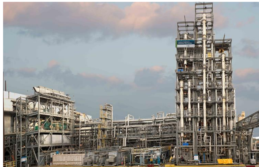
Test Facility for Post-Combustion CO 2 Capture, CO 2 Utilization and DAC Technologies
