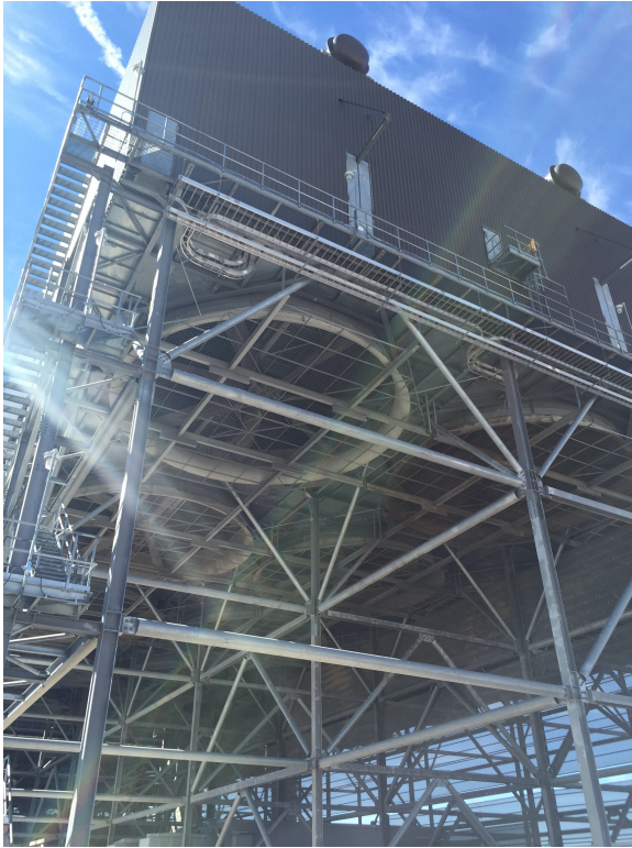
Air-Cooled Condenser (ACC)
