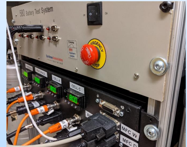
Membrane and cell test stations
