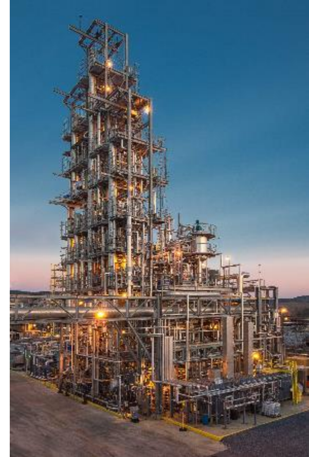
National Carbon Capture Center located at the E.C. Gaston power plant (Wilsonville, Alabama)
