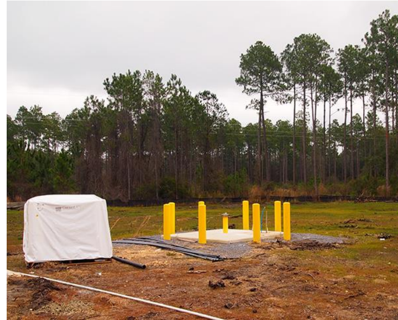
Permanent monitor well installed within 150 ft of injection well is sampled quarterly for water quality impacts associated with injection
