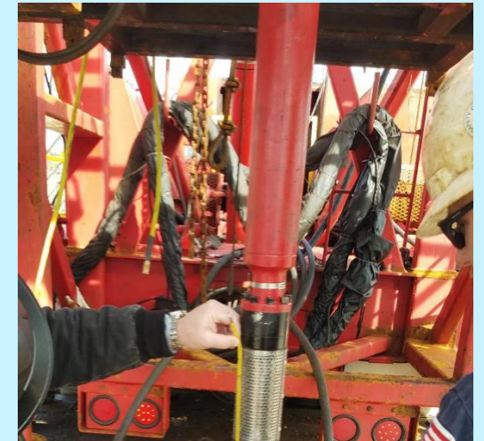
Running and setting electric submersible pump in TEMW-A at 2,022 ft below pad level
