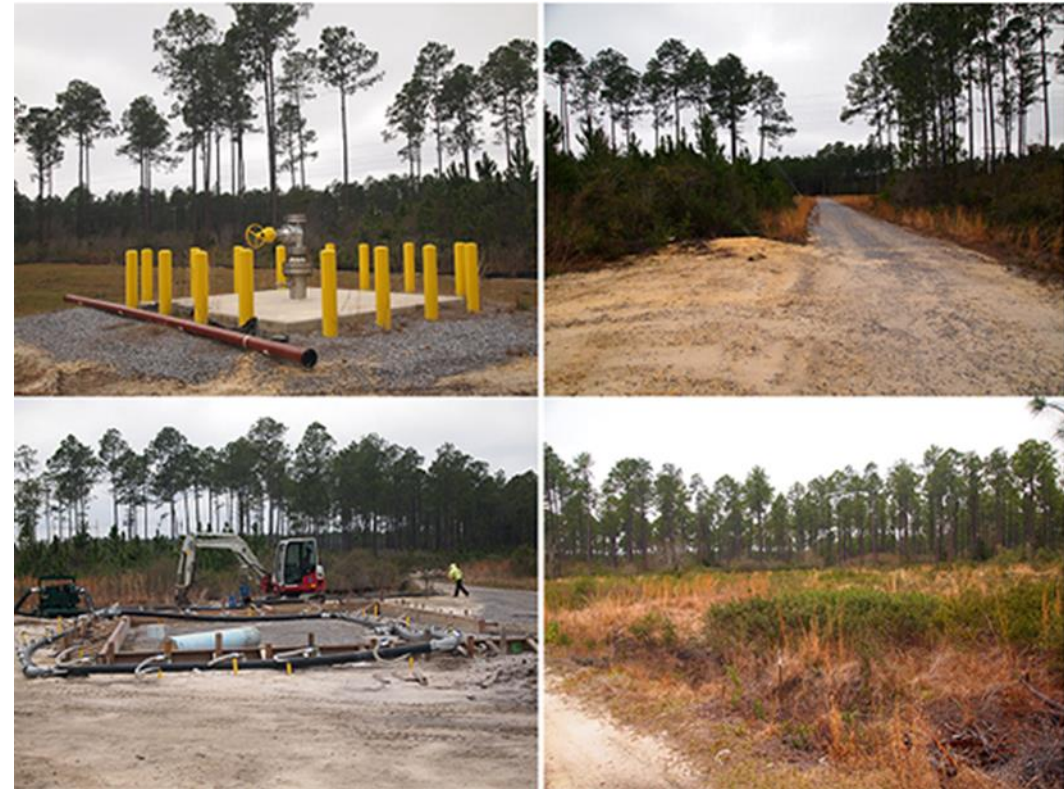
Photographs of existing Gulf Power wellfield. Photos clockwise from upper left: Eocene Injection well EIW-4; graveled access road; pump station under construction; cleared and permitted drilling pad location for future well
