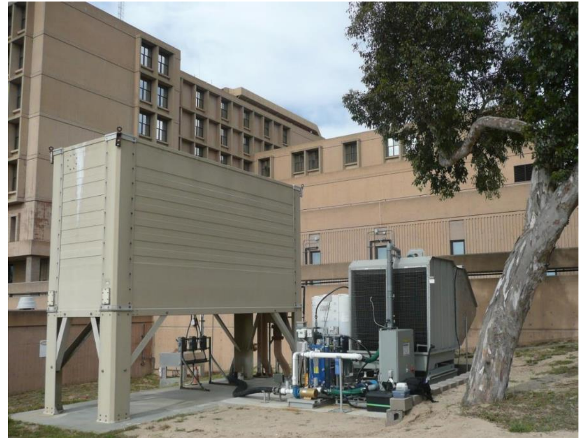
Demonstration site for a hygroscopic cooling system using potable water makeup.
