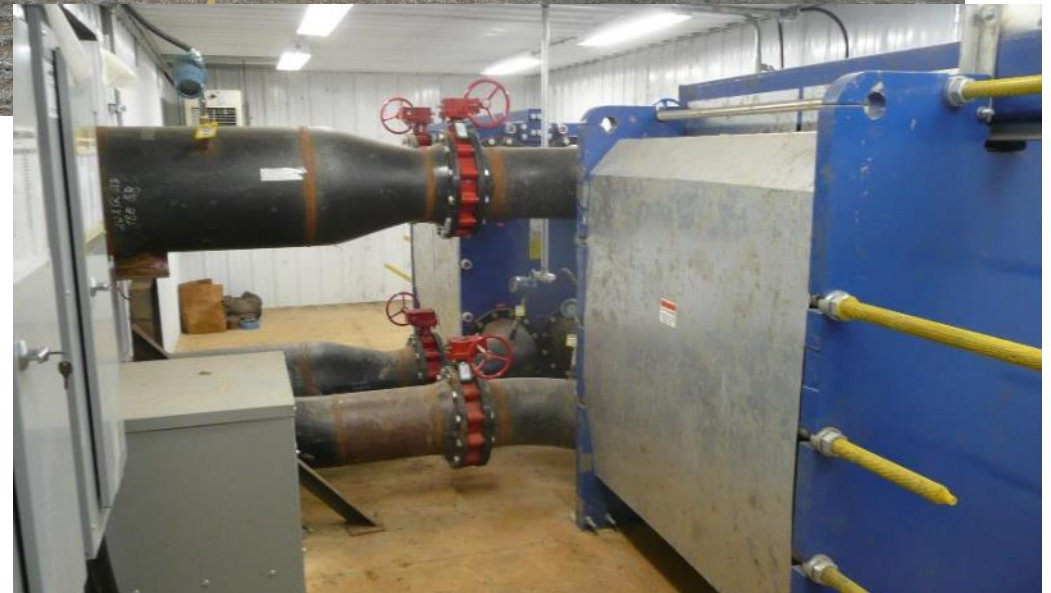
Existing condenser cooling circuit access points at the host site; these connections are planned to be used for the pilot system.
