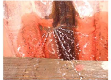
Cracks in transversal direction
