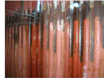
Cracks in longitudinal direction
