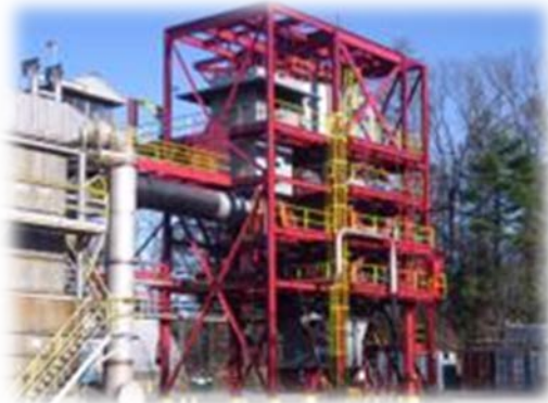
5 MWE Oxycombustion Pilot
