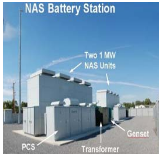
Figure 1: A NAS cell and two MW NAS units. (Photo courtesy of NGK & ESA).
