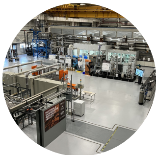
Configurable Facility for Processing and Purifying Solids and Liquids
