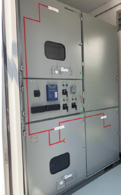
Photo 3.2.2.3c: Inside switchgear enclosure.
