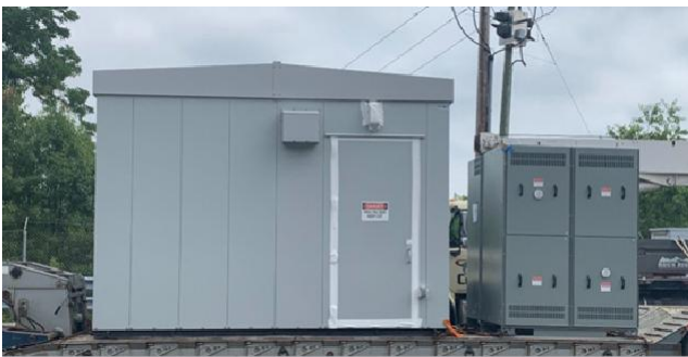
Photo 3.2.2.3b: New switchgear and enclosure.
