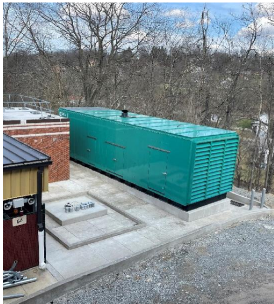
Photo 3.2.2.1.1b: B-83 CAML two-megawatt generator.
