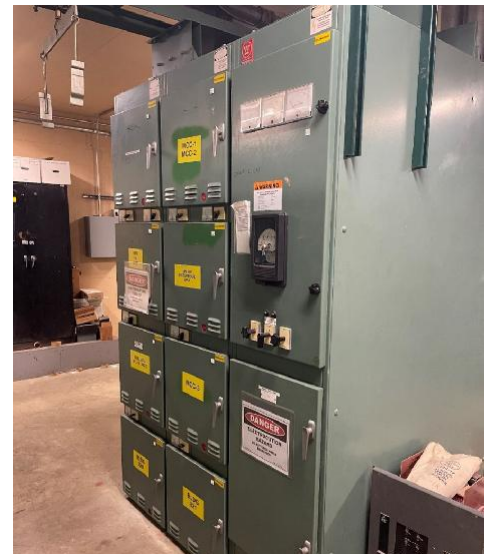
Photo 3.2.2.8a: Outdated switchgear in B-922.
