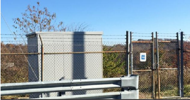
Photo 3.2.2.3a: 920 plateau existing switchgear.
