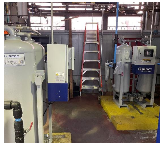
Photo 3.2.2.9b: Newly installed Quincy air dryers.
