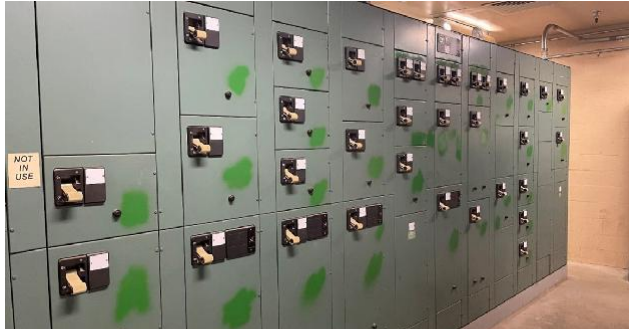
Photo 3.2.2.8a: Outdated and mostly unused MCC equipment in B-922.
