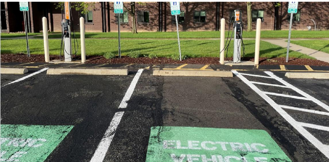
Photo 3.2.2.4: B-83 EV charging station
