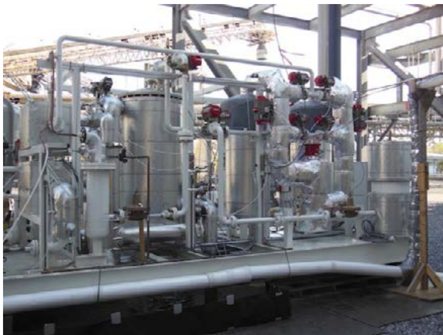
Figure 2: InnoSeptra test skid used for testing at NRG Energy.
