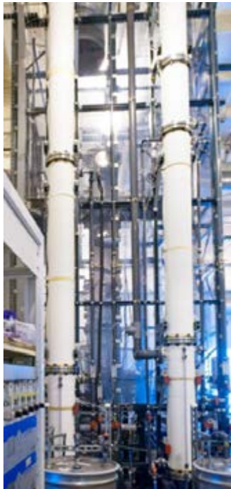
Figure 3: Close-up view of two absorber columns.
