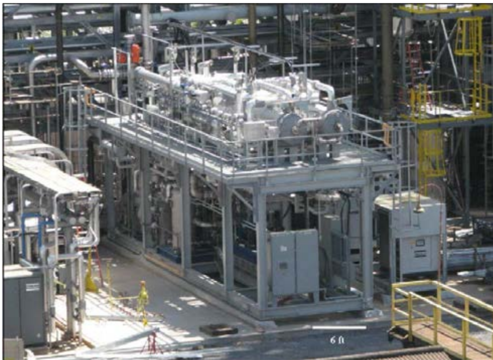
Figure 5: 20-TPD small pilot system installed at NCCC.
