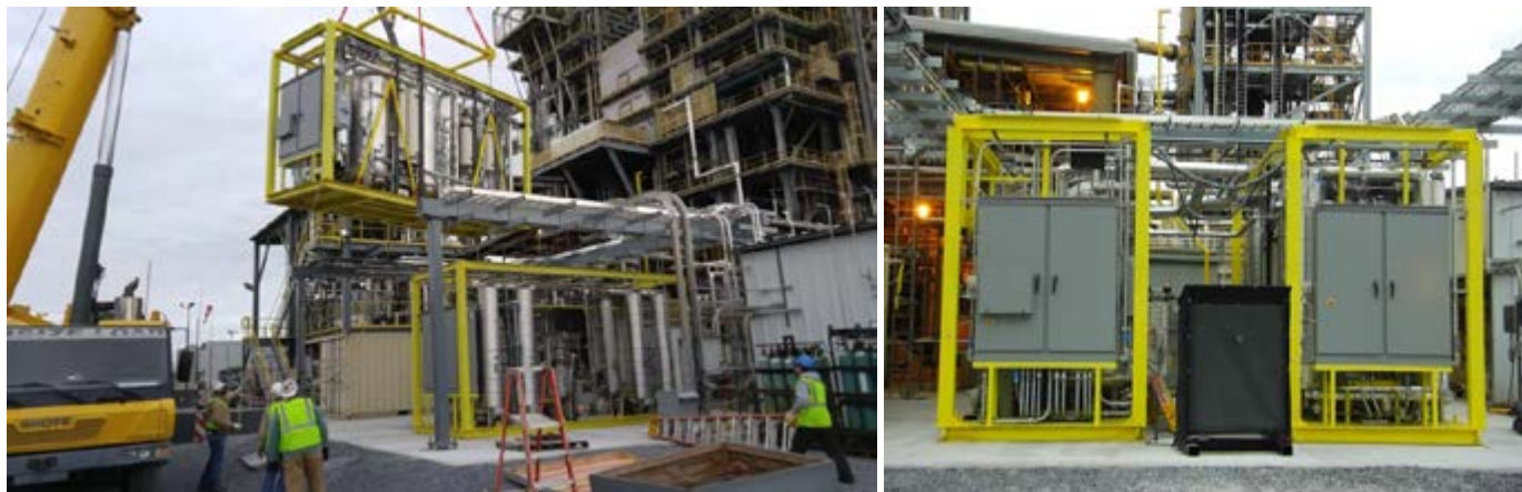
Figure 4: TDA's 0.1-MWe pilot unit installed in the test pad at the NCCC (Wilsonville, Alabama).
