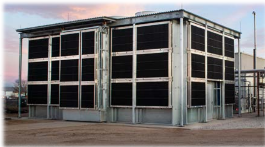
Figure 1: Global Thermostat's kilotonne-scale DAC system as built in Colorado. The larger project module utilizes the same materials, process, and mechanical design as this functional unit.
