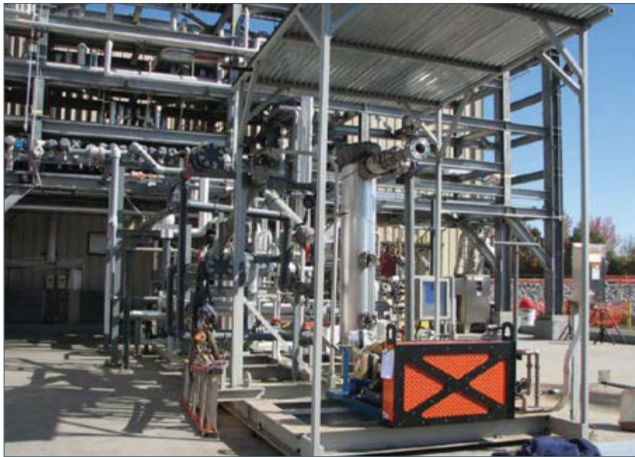
Figure 4: Membrane skid used for 1-TPD bench-scale slipstream testing at NCCC.
