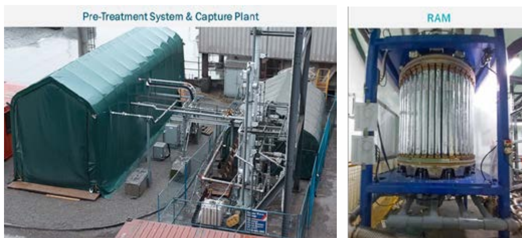
Figure 3: CO 2 MENT field Unit (1 TPD) at a Lafarge cement plant in Richmond BC showing the pre-treatment system and capture plant (left) and the RAM showing the beds (right).
