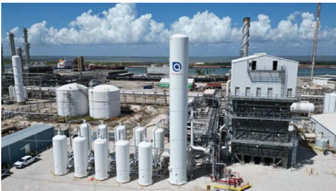
Figure 2: Air Liquide SMR plant host site.
