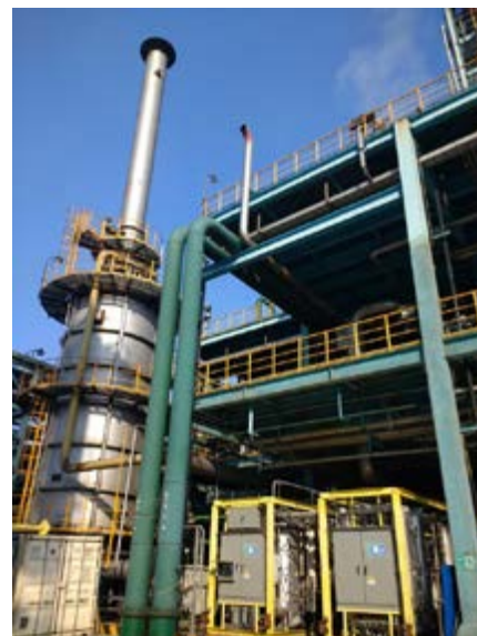
Figure 5: Field test units at Sinopec, China.
