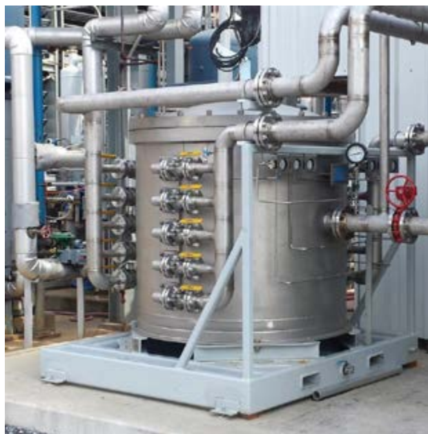
Figure 6: Prototype plate-and-frame module during testing at NCCC.
