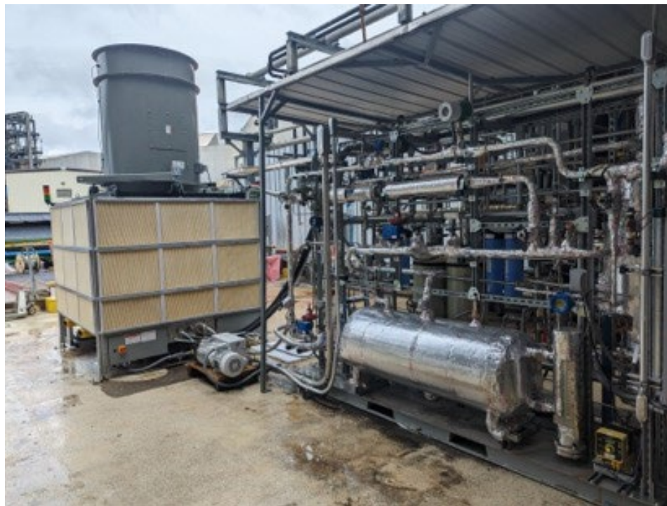
Figure 2: DAC and heat treatment skid installed at the NCCC.
