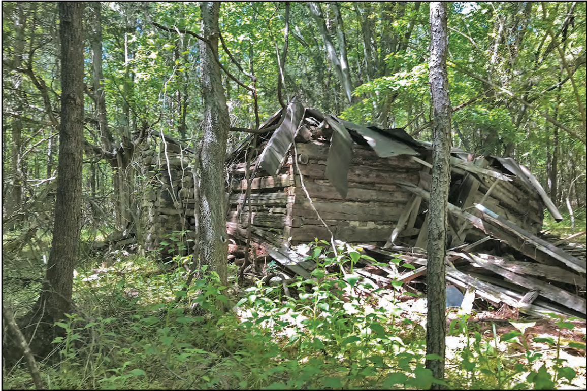
PLATE 1: Collapsed Cabin at Site 44PY0394, Facing Northwest
