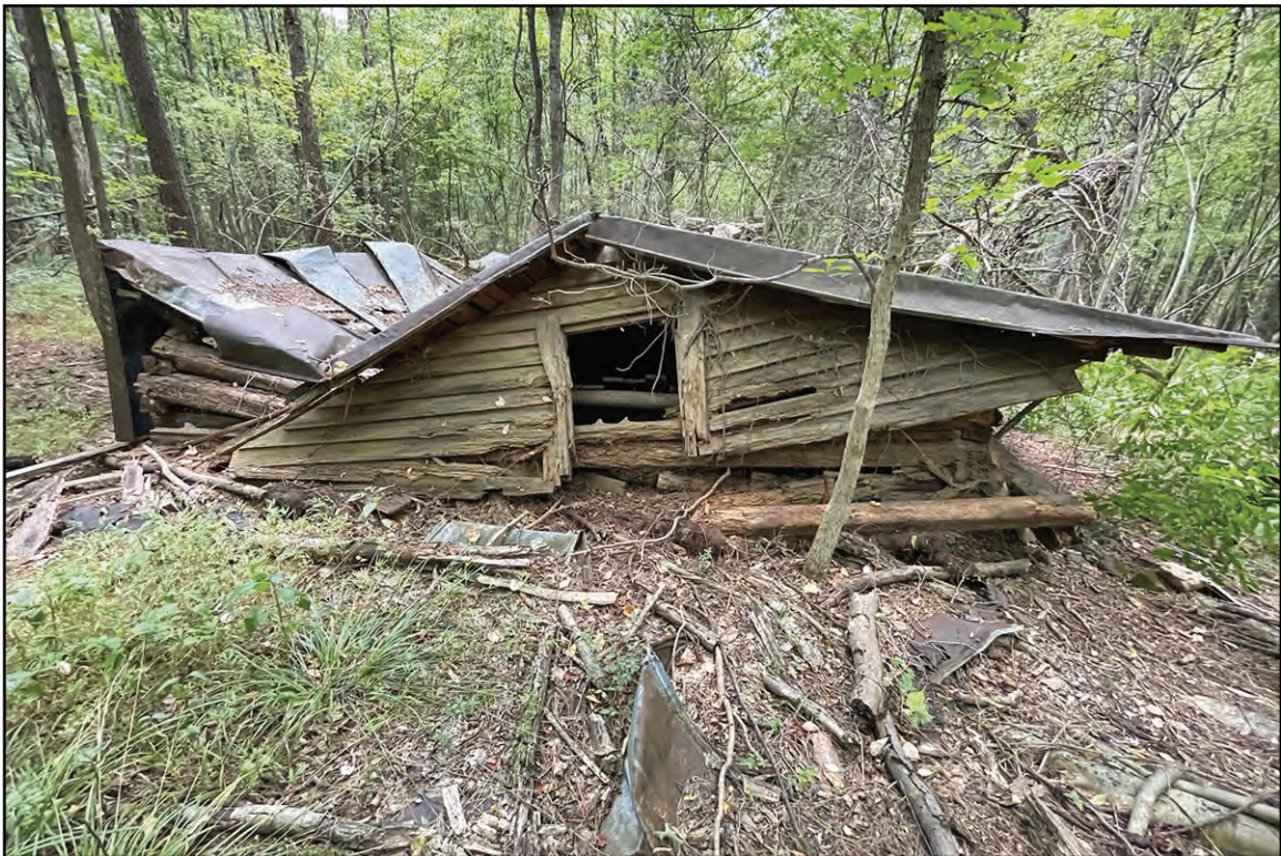
PLATE 2: Collapsed Cabin at Site 44PY0394, Facing North
