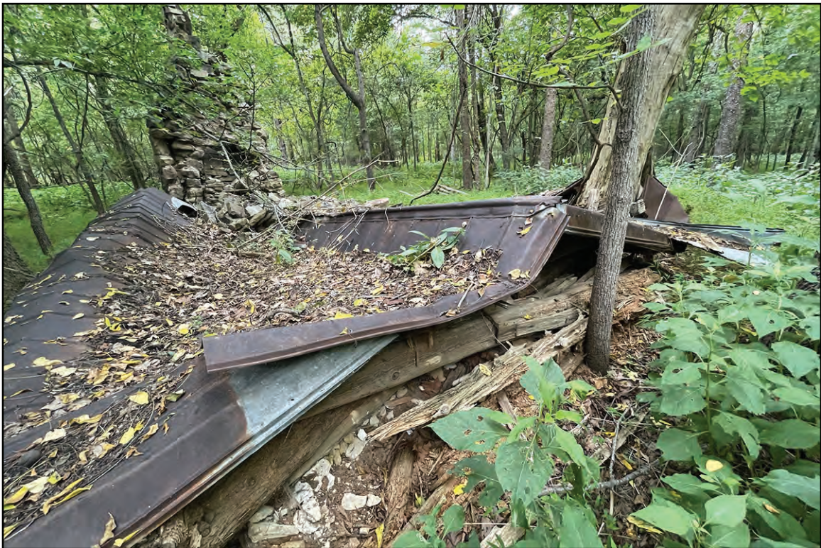
PLATE 5: Collapsed Cabin at Site 44PY0398, Facing Northwest
