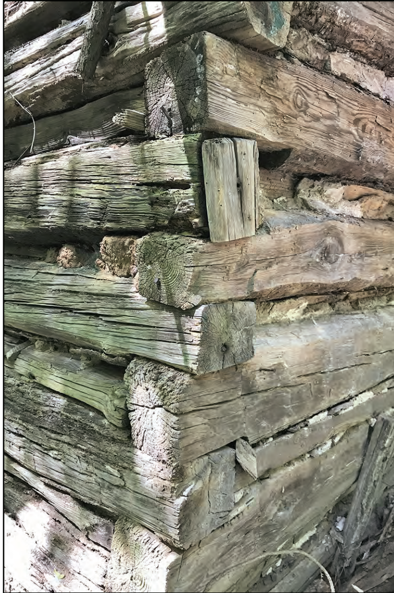
PLATE 3: Northwest Corner of Collapsed Cabin at Site 44PY0394
