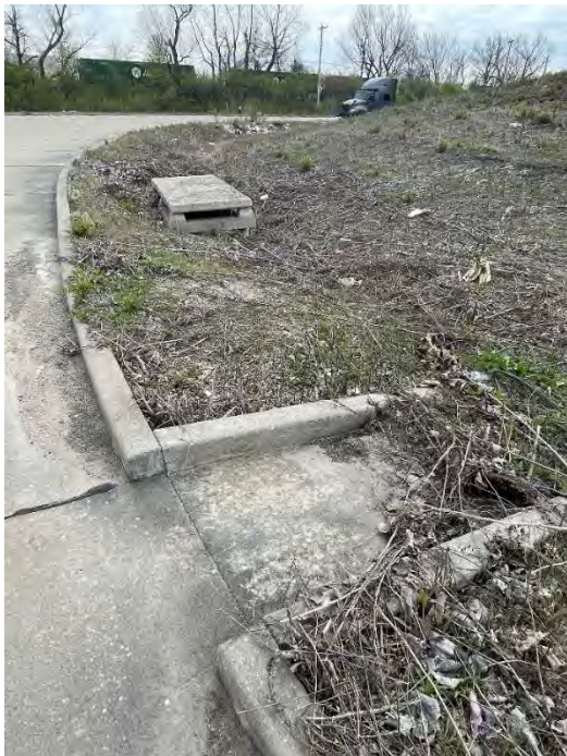
View of the catch basin, located north of the mound along the "L" shaped road.
