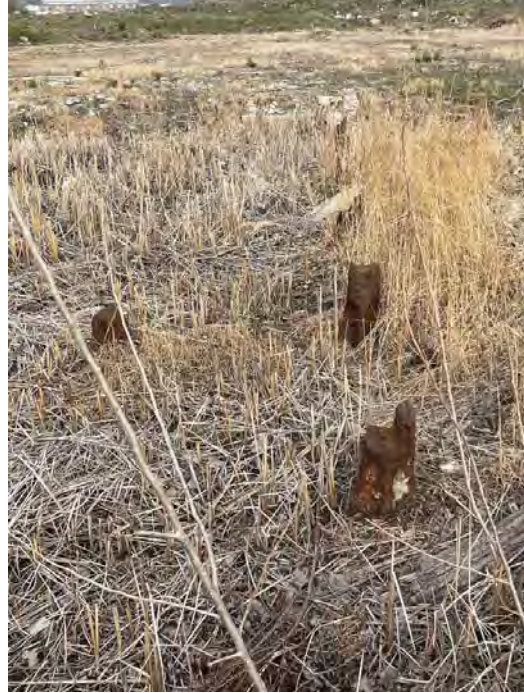
View of rusted metal stick-ups located in the pit located near the center of the proposed project site.
