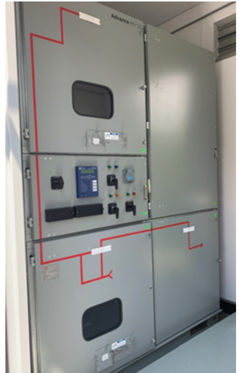
Photo 3.2.2g: Inside of the switchgear enclosure.
