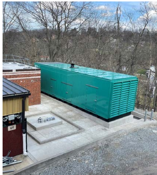
Photo 3.2.2b: B-83 CDAML – a new two-megawatt generator.
