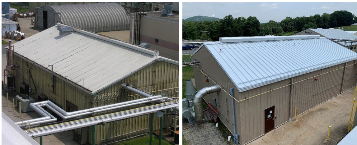
Photo 3.3.2a: Before (left) and after (right) showing the new exterior and roof of B-13 featuring added horizontal lifeline fall protection
